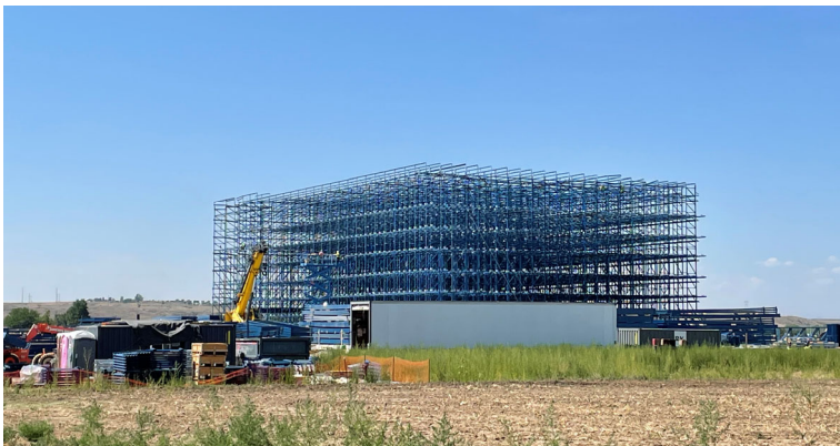
Great Western Industrial Park 13th Filing L3 (Ceti Alpha Cold Storage Facility)
